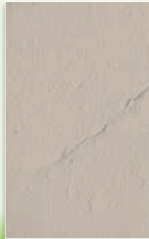
Medium cracks (1 to 2 mm)
